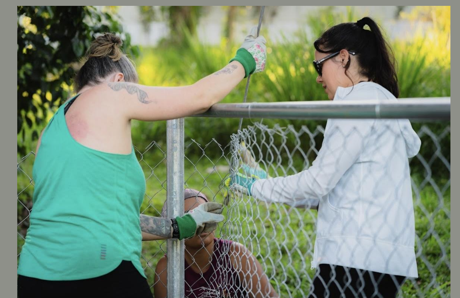
Figure 3: OSU students and volunteers constructing a fence around the community garden (Photo by J. Jordan)
