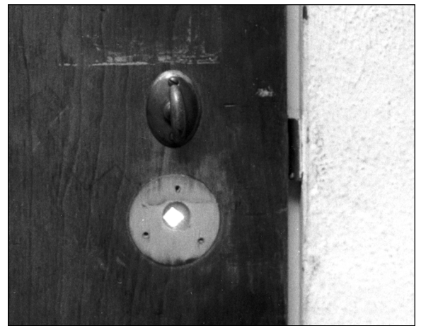
Figure 11. Minor items, such as a door knob hole, can cause major problems. This can result in the loss of truckloads of food production.
